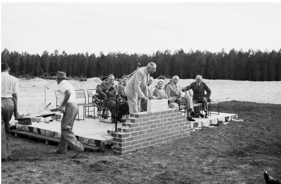
Hon Ernest Knight (EK) Hoare MLA Minister for Agriculture laying the foundation stone at the Department of Agriculture South Perth office, 1956. (Photo credit: DPIRD)
