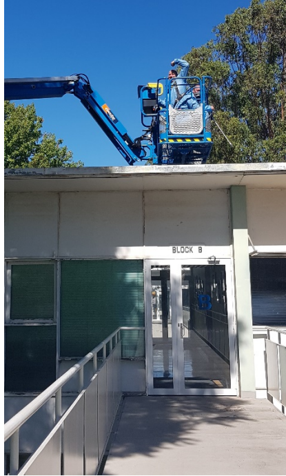
Asbestos roofs at DPIRD South Perth get painted with Acrylic coating aiming to stabilise airborne asbestos fibre contamination.
